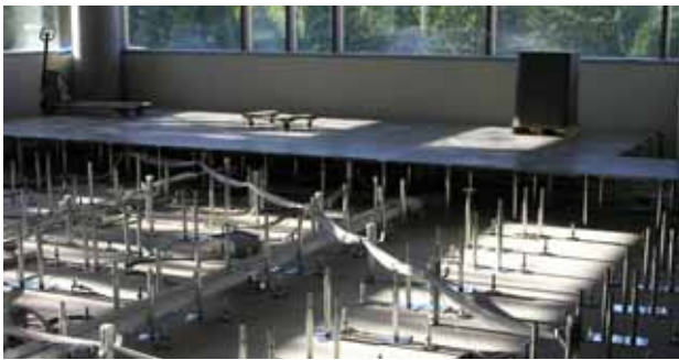
Office floors raised for under-floor concealing of mechanicals, electrical, and HVAC
